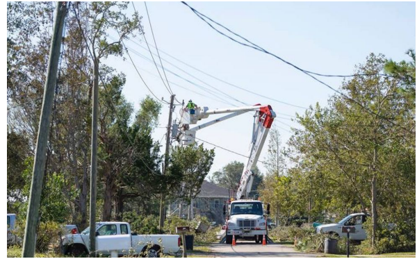
Figure 3: Damaged Powerlines after Hurricane Zeta (5)
